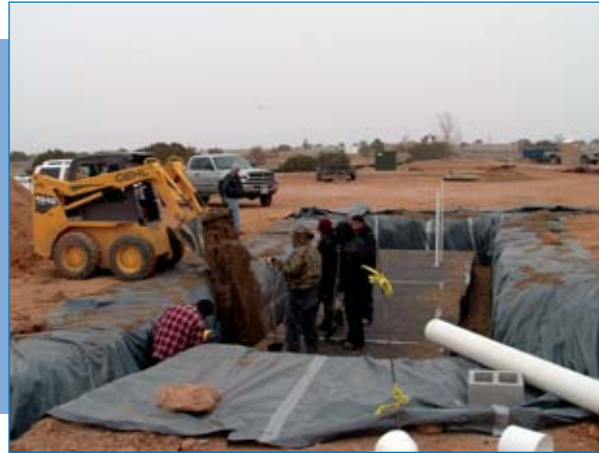
Sand and gravel backfill mixture is used between modular tanks and impermeable liner for structural support and to provide a means of underground purification for water being held. The liner creates an artificial aquifer environment from which water is extracted from the modular tanks.
