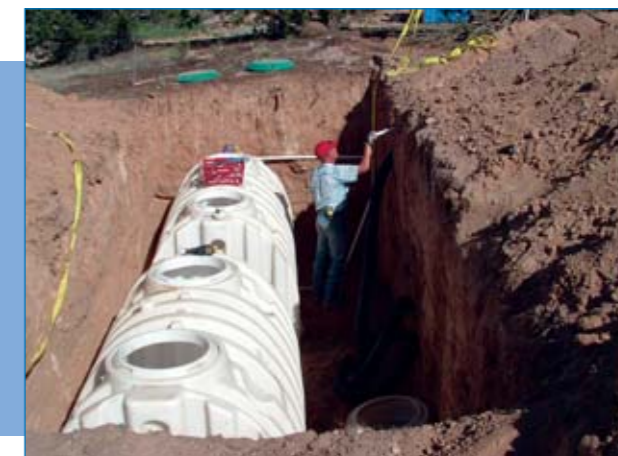
Two 1200-gallon holding tanks connected to create 2400 gallon capacity for new custom home.
