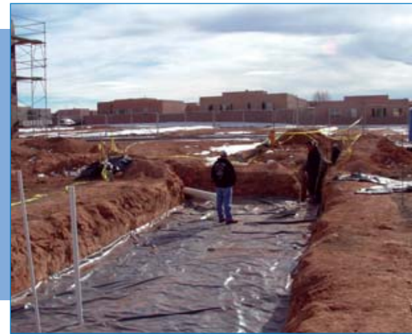
Large rain-harvesting system completed, ready for backfill and final grading above tank.
