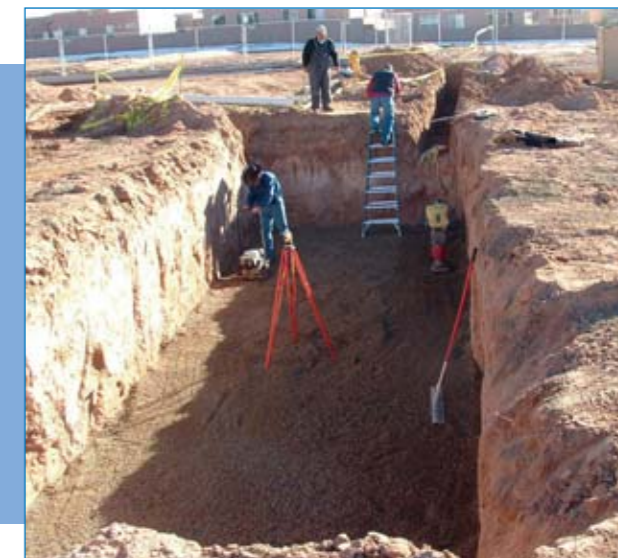
Hole preparation for large modular rain-harvesting system. Excavation should be level and compact for modular designs.
